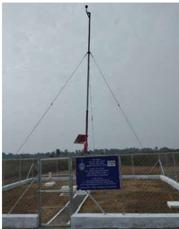
Fig. 3.29. Weather station installed at IARI-Jharkhand
